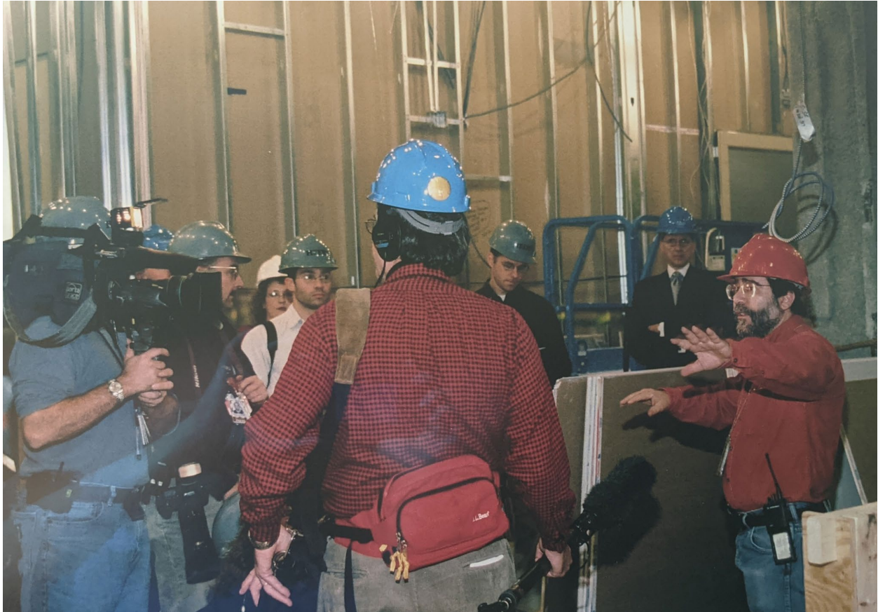
Rick Blondo (wearing a red construction helmet) discussing the National Archives renovation project to the press, circa 2002.
